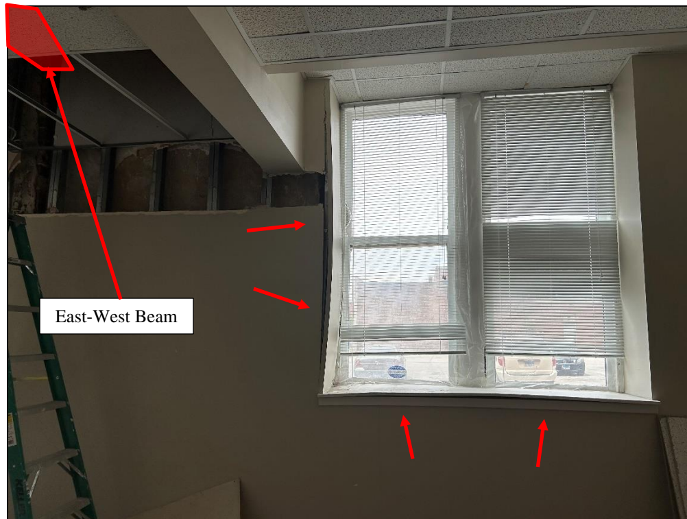
Photo 3 – Excessive Downward Pressure on Finishes
