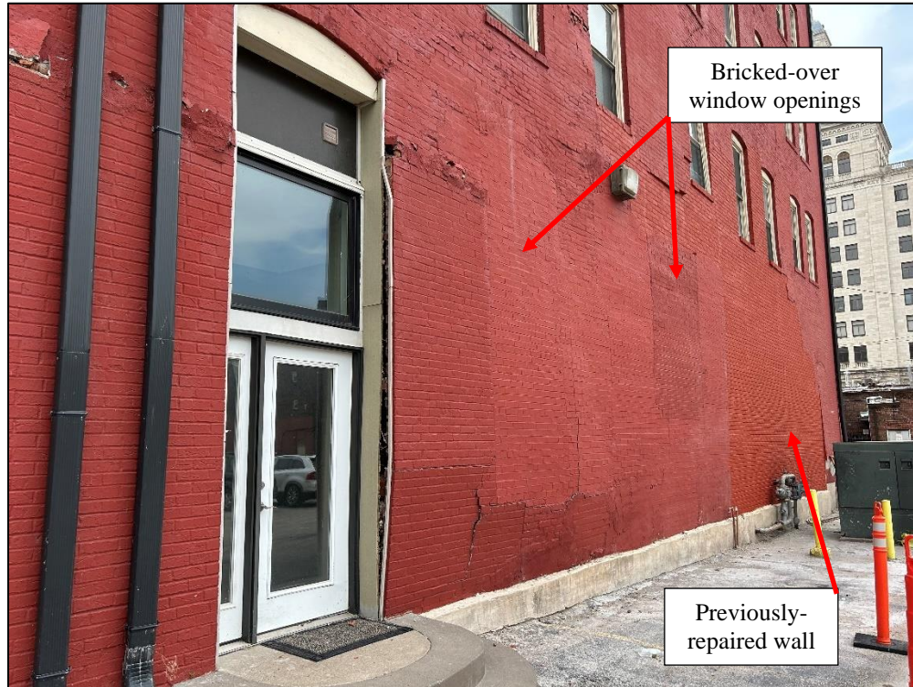
Photo 1 – Clay Brick Façade pulling away from Substrate
